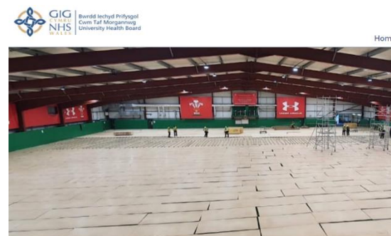
Field Hospital takes shape – Work to increase bed capacity at Cwm Taf Morgannwg UHB
